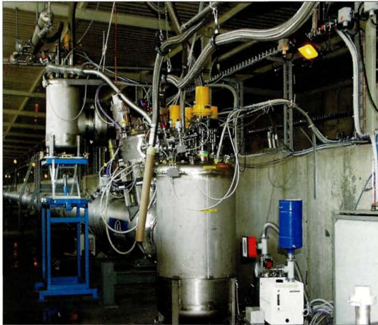
One of three 112 m test cells for CERN's Large Hadron Collider (LHC) cryogenic distribution line (QRL). End-boxes close the interconnections that will eventually join QRL cells together and the service modules that will connect the QRL to the LHC's magnet cryostats. One service module is visible here at the near end of the test cell.
